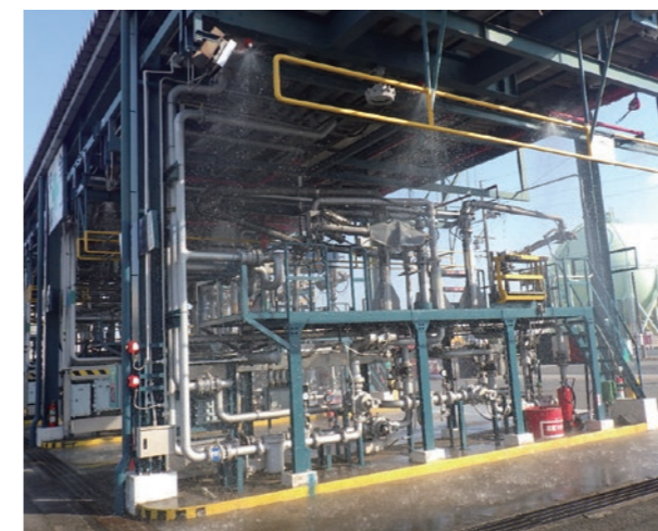
Spraying from the foam-water sprinkler head of the tanker truck loading dock
